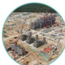
Cracker area aerial view
