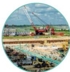
Cooling water tower and pipe bridge
